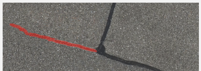
Figure 5: The automatically detected cracks are highlighted in red and supplemented with information on length and severity of the defect (see next section).
